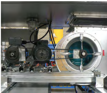
Run and Standby Motor
